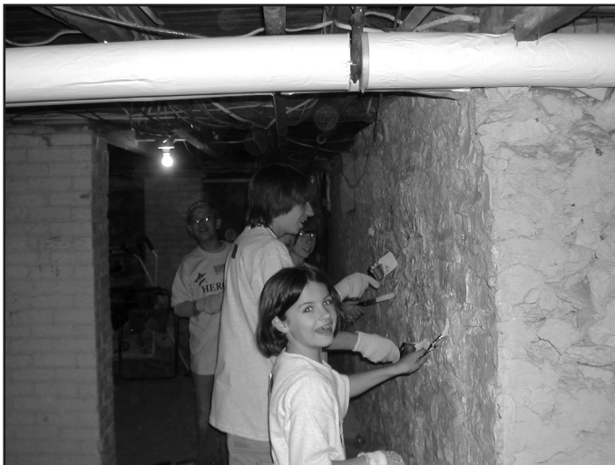
Youth volunteers from Rebuilding Together Saratoga County (RTSC) painting the Vet House basement
